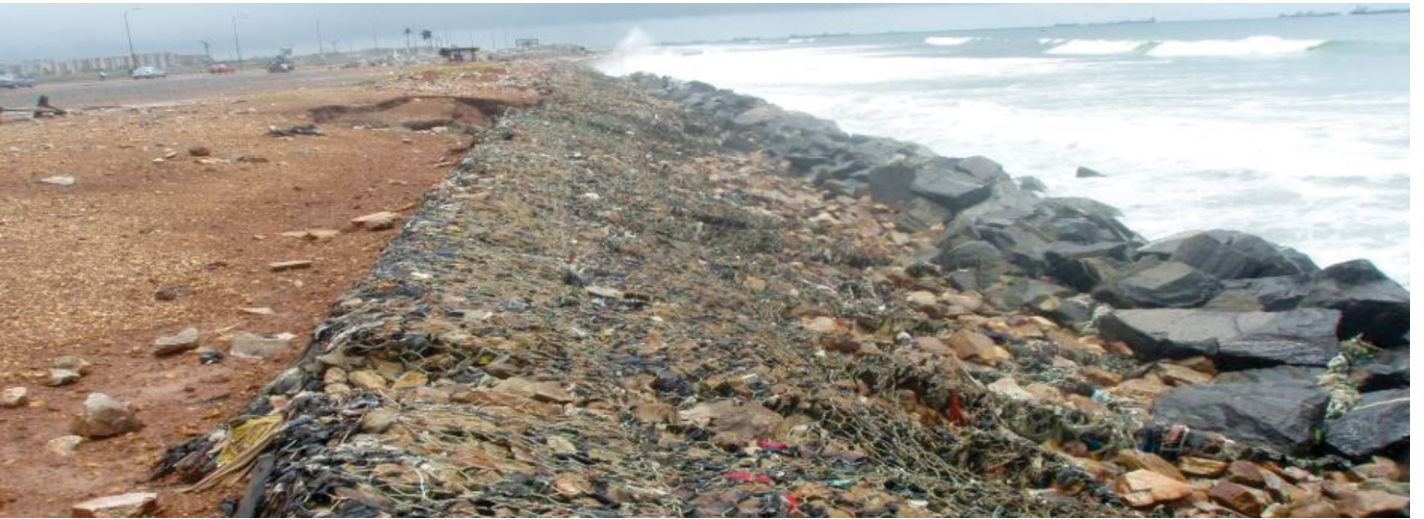
Plate 3: Beach nourishment, gabion and riprap at Sakumono beach. Beach nourishment shows signs of erosion
